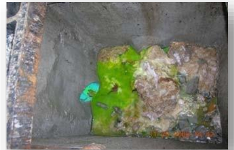
Service station toilet connected to a storm water catchbasin by accident
